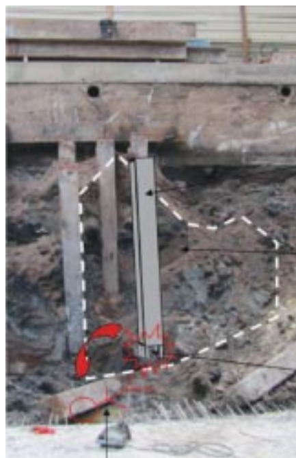
Deceased hit by collapsed RC pile
