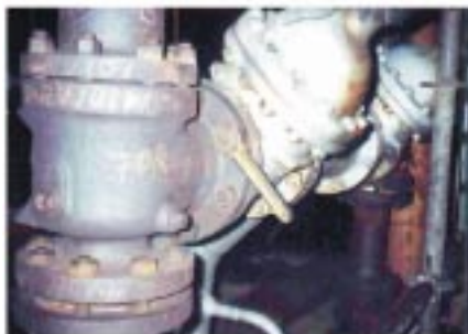
Close-up view of the relief valve which leaked.
