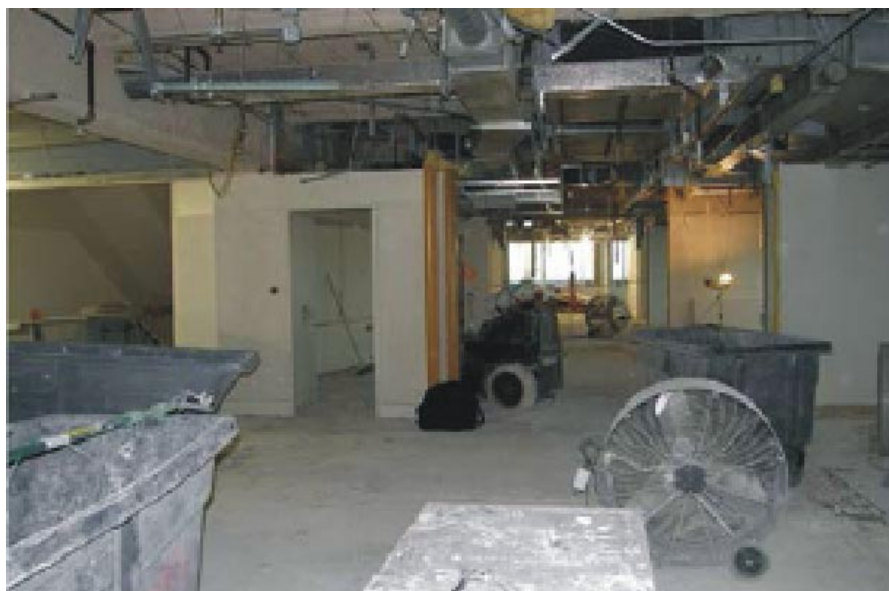
Running just one propane-powered machine in a poorly ventilated space can lead to carbon monoxide poisoning, even in larger spaces like this one.
